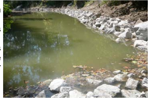
Peaked stone riprap provides erosion protection.
