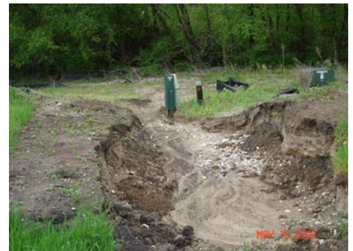
Gully caused by excessive runoff. Notice high voltage utility box on right side
