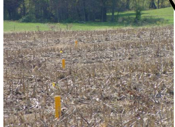
The completed terrace system will collect stormwater runoff and safely convey the water to a stream through underground tile lines.
