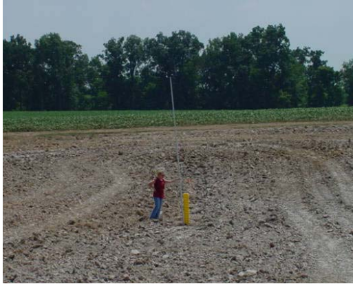
District employees survey the elevation of an underground tile inlet which will allow water to safely escape from a terrace system
