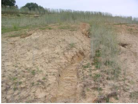
Erosion Taking Place Before Erosion Blanket Installed
