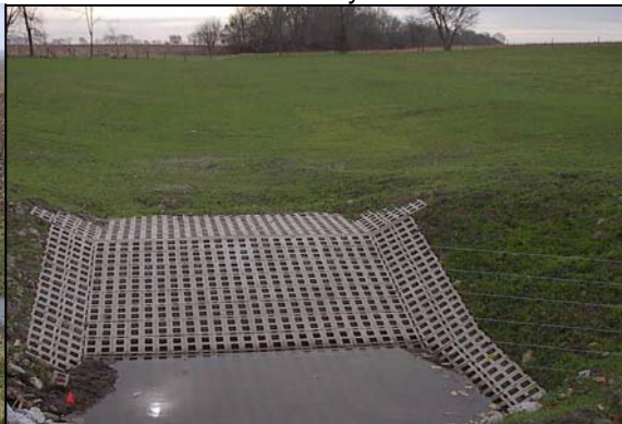
This picture is of a block chute at the end of a waterway.
