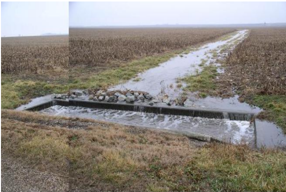
This is a Drop Box Structure at the end of a waterway. The amount of water you see is from a ¼ inch rain.
