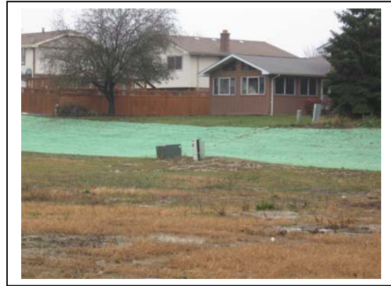
After: Completed treatment of disturbed area after application of excelsior blanket material
